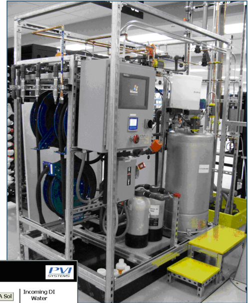
Clean & Fill System at IBM's Poughkeepsie, NY production facility.
