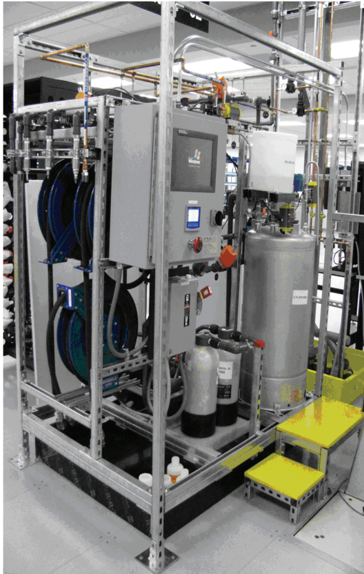
Clean and Fill System at IBM's Poughkeepsie, NY production facility
